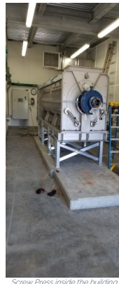
Screw Press inside the building
